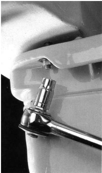
13 Tighten nuts with ratchet wrench until tank is snug. Use caution when tightening nuts: most toilet tanks rest on the spud washer, not directly on the toilet base.
