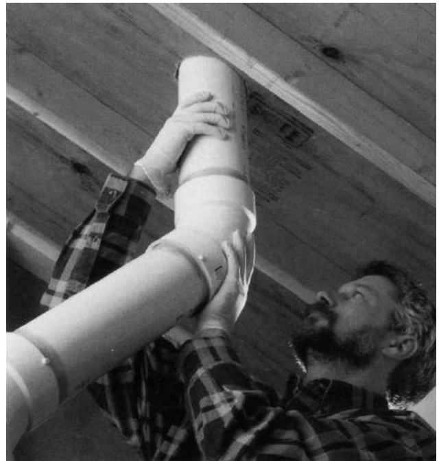
16 Finish the waste-vent stack installation by using 45° elbows and straight lengths of pipe to extend the stack through the same roof opening used by the old vent stack. The new stack should extend at least 1 ft. through the roof, but no more than 2 ft.
