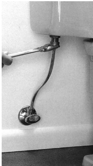
14 Attach the water supply tube to the ballcock tailpiece with an adjustable wrench (page 216). Turn on the water and test toilet. Tighten tank bolts and water connections, if necessary.
